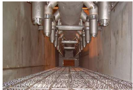
Internal Distribution Water Nozzles and Packing Arrangement
